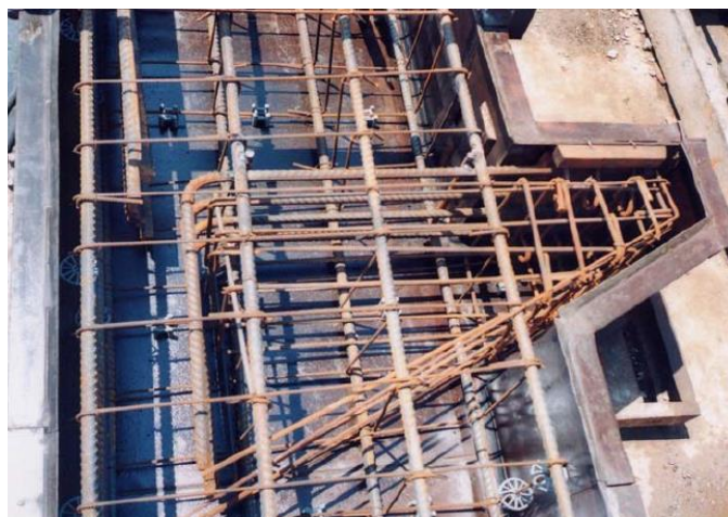
Figura 4. Acero de refuerzo de columna y ménsula (FÉDÉRATION INTERNATIONALE DU BÉTON, (FIB), Structural Connections for Precast Concrete Buildings, February 2008).
