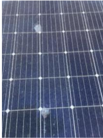
Fig. 5. Panel solar quebrado
