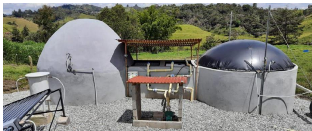
Figure 6. UASB reactor from porciCES. An experimental farm of CES University.
