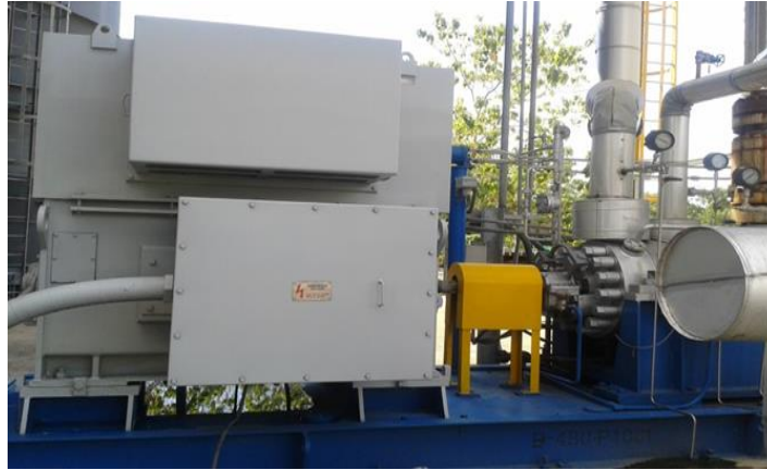
Figura 42. Motor de bomba FEED WATER.
